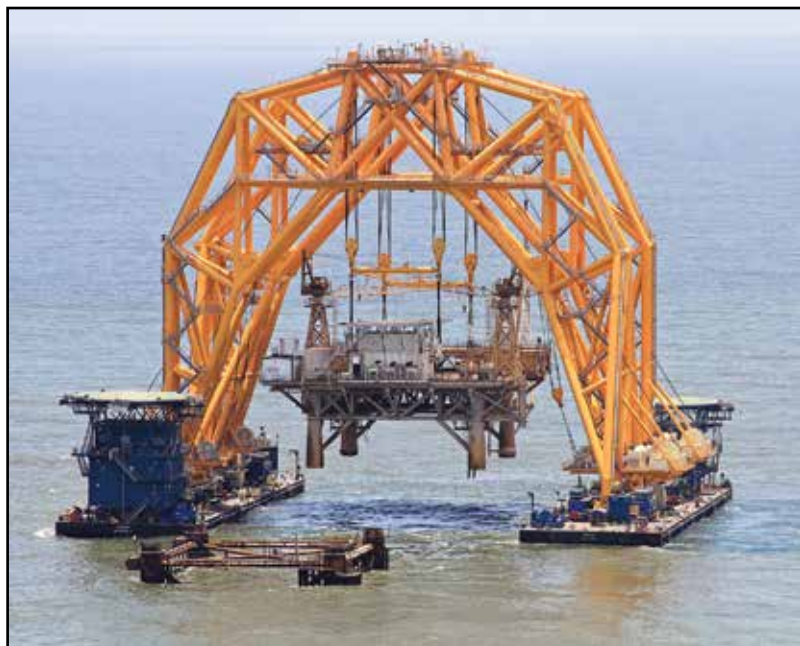
The VB 10,000 is a heavy-lift twin-gantry catamaran used to remove shallow water drill platforms in the Gulf of Mexico. The VB 10,000 is used in conjunction with the VersaCutter, a subsea steel cutting tool that can cut platform anchor pipes 15 feet below the mudline.
